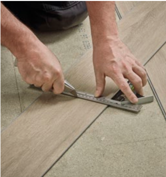
1. Using a knife and a straight edge, measure the first plank to no smaller than the width of the plank.
